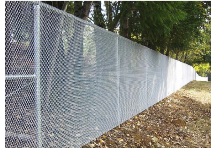
Photo A01 Example of chain link security fence with mini-mesh
